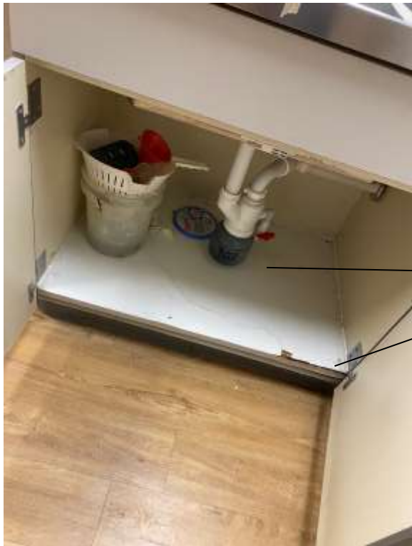
Photo #2 Beneath Northeast sink – Damaged and deteriorated Veneer. Sample 25903-02-0106B & 25903-02-0107A taken from cabinet on veneer and exposed wood.
