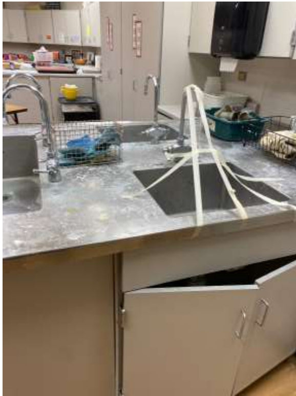
Photo #1 Northeast sink – Issue with water damage
