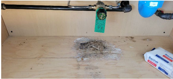
Photo 1 - Below a sink in room 710, during the assessment.
